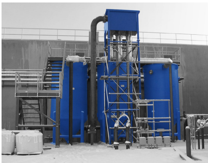
0.75 MGD (33 L/s) Centra-flo™ installation in New York
